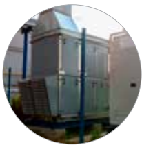
Air handling units
