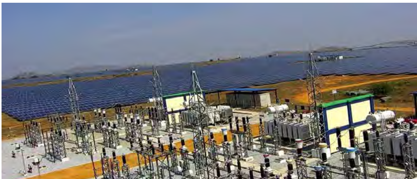
REC financed 300 MW solar power project of Avaada Energy Private Limited in Pavagada Solar Park, Karnataka
