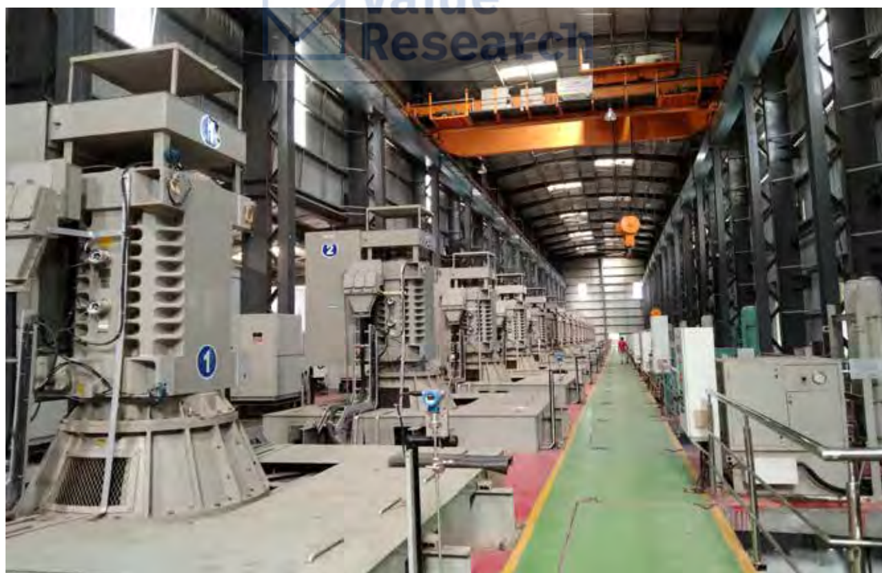
Pump-house of Purushothapatnam Lift Irrigation Scheme Stage-I at Andhra Pradesh, financed by REC
