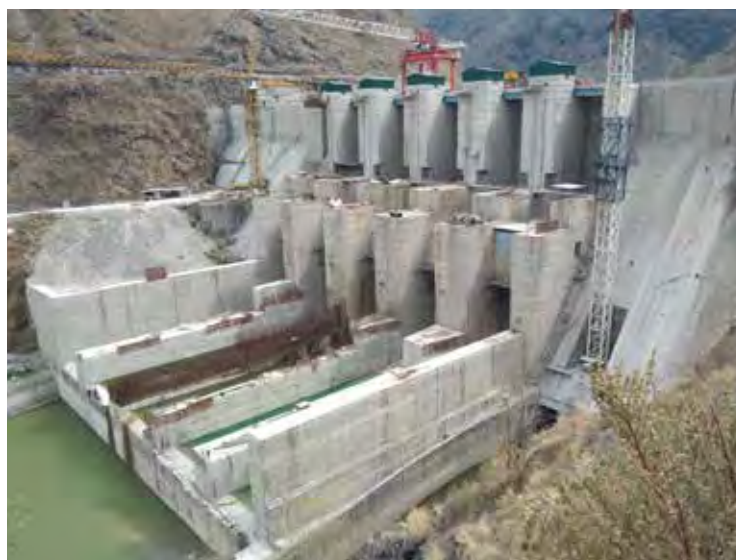
REC financed 2x60 MW Vyasi Hydro-electric Project in Dehradun, Uttarakhand
