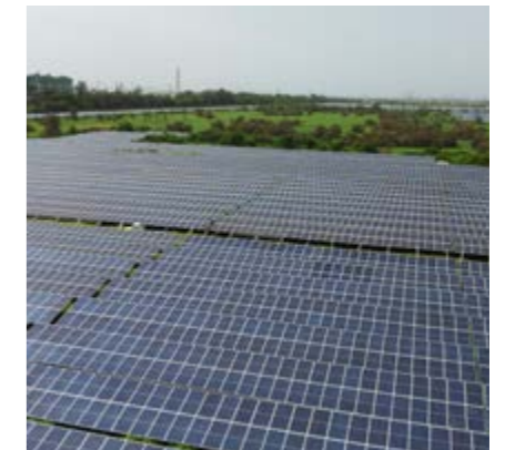
We deployed a 56 MW solar plant, utilising both floating and ground-mounted installations, in Kawas, Gujarat.
