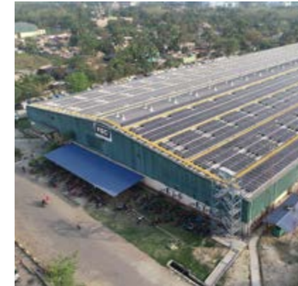
We also implemented Eastern INDIA'S LARGEST ROOFTOP solar project of 2.1 MW for The Keventers, West Bengal.
