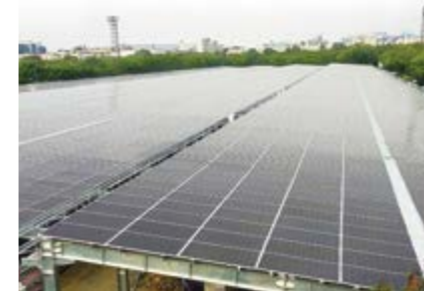
We commissioned a 5 MW carport project for Maruti Udyog Limited.
