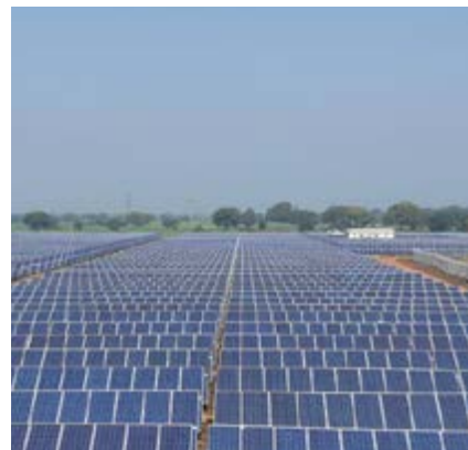
We commissioned a 20 MW project for BEL in Itarsi, Madhya Pradesh.
