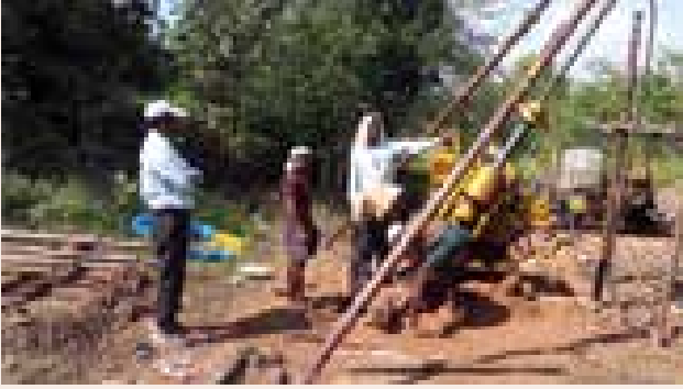
Drilling work for inclined borehole in progress for the proposed tunnel of Pendlimarri-Rayachoti section (Phase-II)
