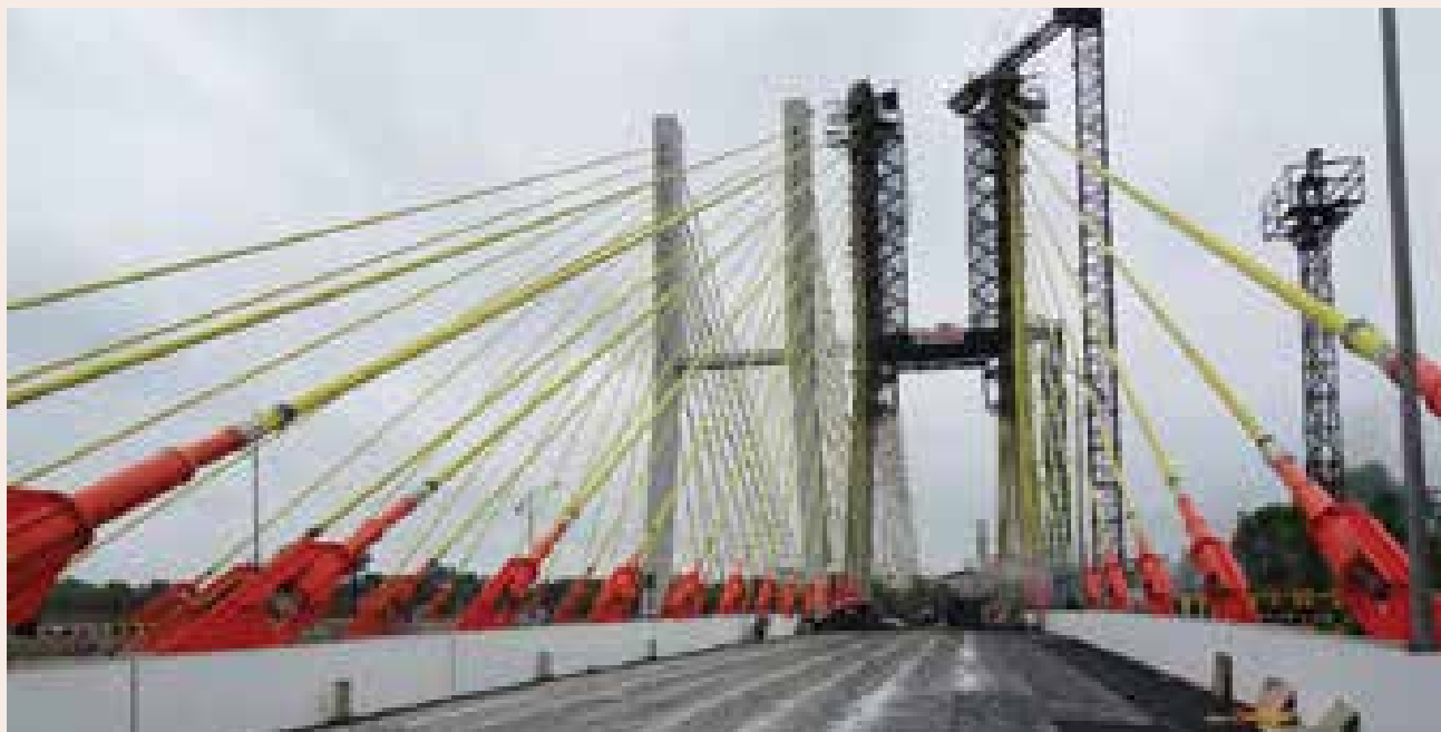
Engineering the design and construction of Six Lane Cable Stayed Bridge along with Approaches near Santra Market, Nagpur
