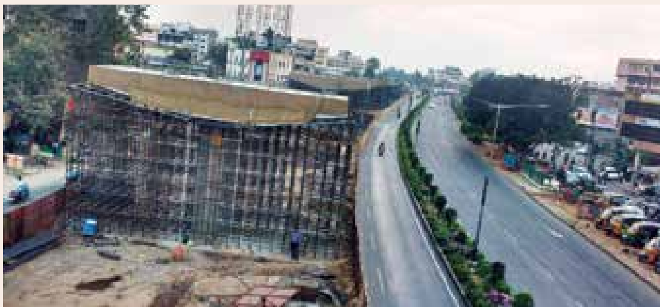
Flyover construction at Benz Circle on Vijaywada-Machilipatnam Section of NH-9 in Andhra Pradesh
