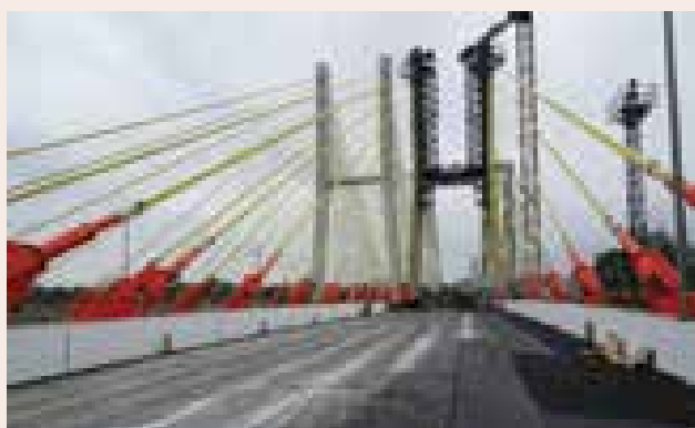
Engineering the design and construction of Six Lane Cable Stayed Bridge along with Approaches near Santra Market, Nagpur.jpg
